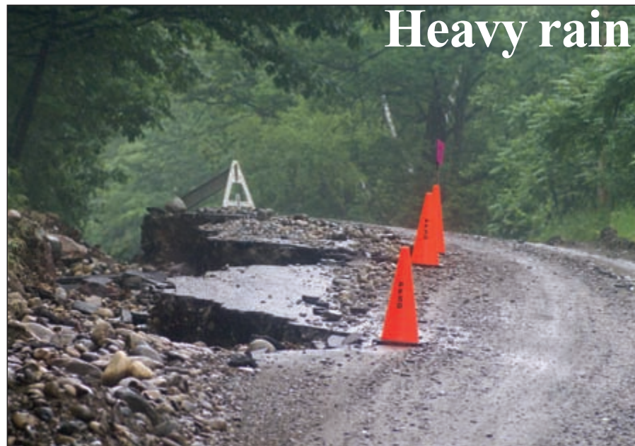
Sections of Wheeler Hill Road are almost completely washed out from the heavier than usual rains of late. The Phillips road crew will be challenged over the next few weeks to repair them. (David Hart photo)
